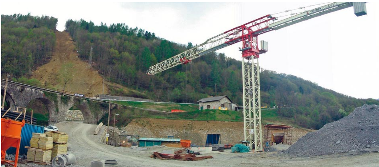
Construction of the powerhouse shaft, in the background soil excavation for the penstock
