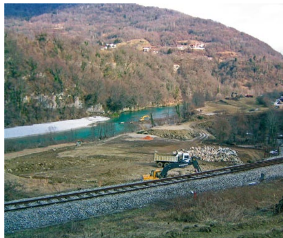
Location of the powerhouse shaft on the terrace of the Soča River
