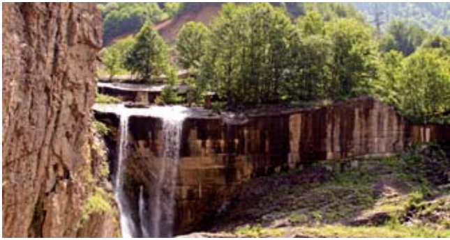
Linkes Widerlager - Alte Betonblöcke in der Mauerfundation Left dam abutment - old concrete structures in the foundation
