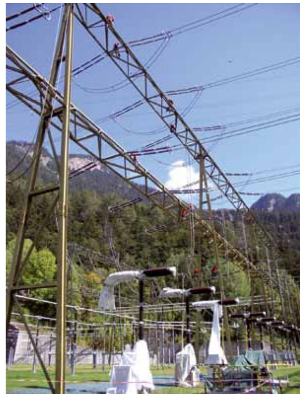
Corrosion protection of the steel structure (right) Installation of the new SF6 instrument transformers (left)
