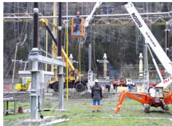
Installation of new disconnecting switches (right) Dismantling of the old disconnecting switches (left)
