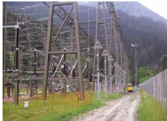
Access road for installation of surge arresters (right) Installation of relay house (left)
