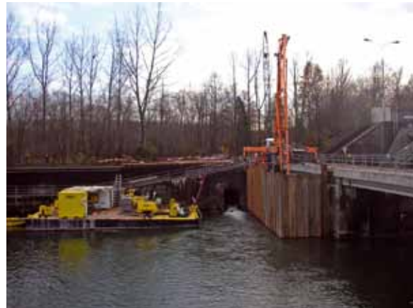
Works on the sheet pile wall in the weir opening no. 3 (right), Hydraulic model test with rehabilitated stilling basin (left)
