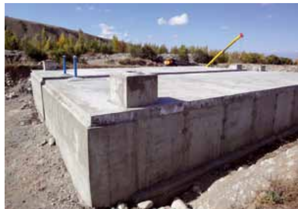
New clear water reservoirs (2 x 1,500 m 3 ) (right) Rehabilitation of groundwater wells (left)
