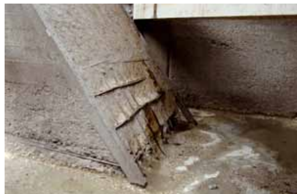
Damage to the baffle block (right) The Flumenthal run-of-river plant (left)
